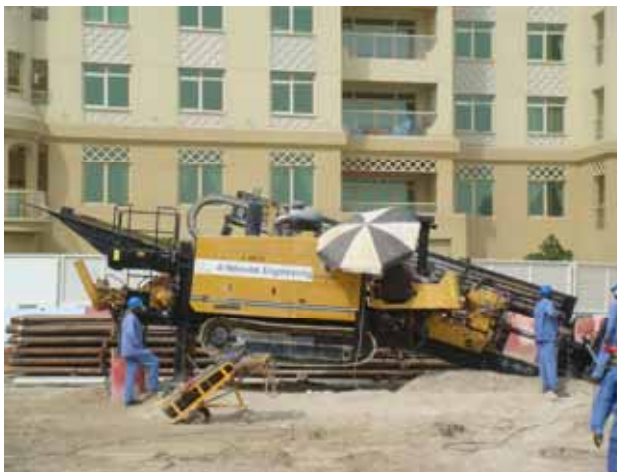
The Vermeer NAVIGATOR D100x120 drilling rig used for the smaller diameter boring work.
